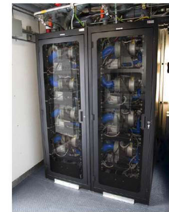
(2) HyPM™-R120 installed within sea container (240 kW gross )
